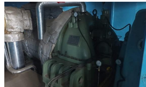
Gambar 2. Mesin Steam turbine
